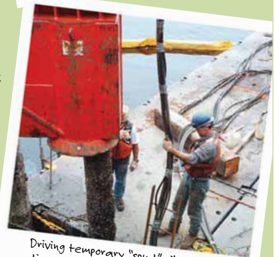
Turner's teams replaced 760 rotted wood "toothpick" piles with 270 Duplex-coated steel piles on Pier 59
